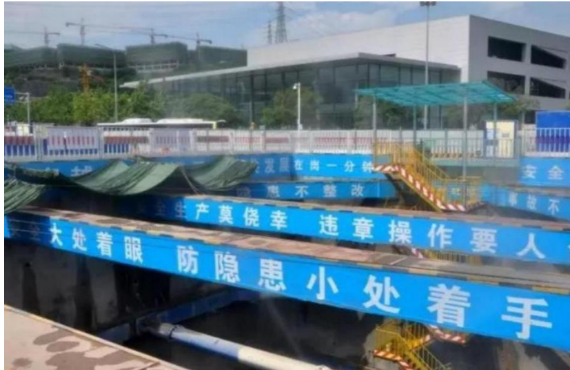
Fig. 12 3TBM Launch Shaft Spray System
