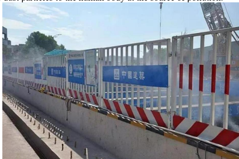
Fig. 13 Water Mist Dust Suppression System
