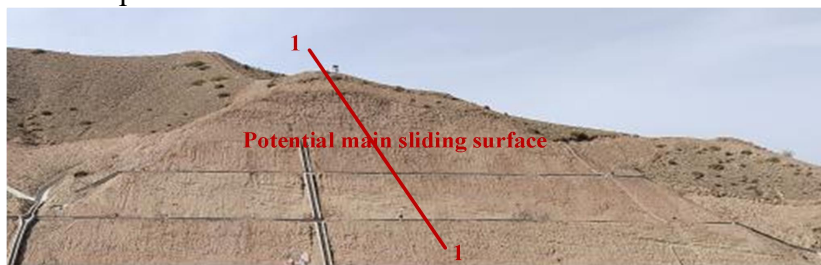
Fig. 1 Potential main sliding surface of the slope
