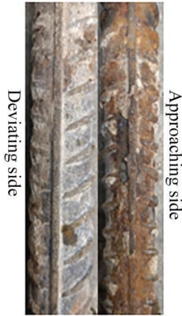
Fig. 2 Corroded steel bars in the specimen
